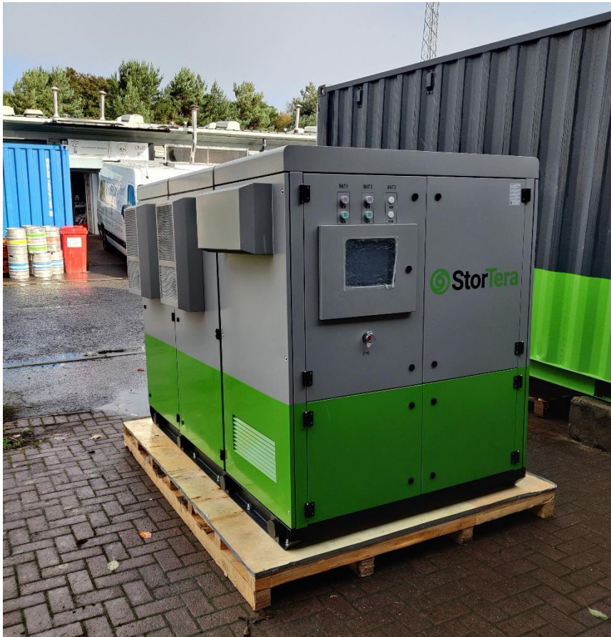
Figure 3: Example photo of small battery enclosure
